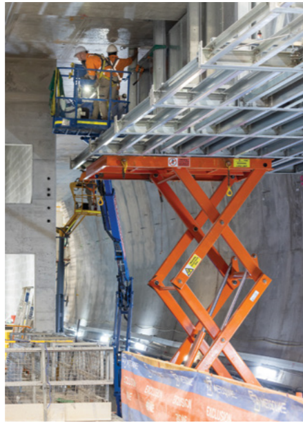
At the 2022 Lendlease Australian Supplier Awards A.G. Coombs was recognised with the Safety Award for the innovative solution developed for the design, manufacture, supply and installation of over track exhaust modules.
